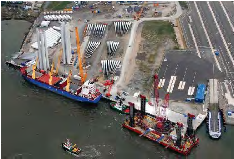
Figure 7.1: Port of Mostyn Construction Base for Burbo Bank Offshore Wind Project (UK) 85
